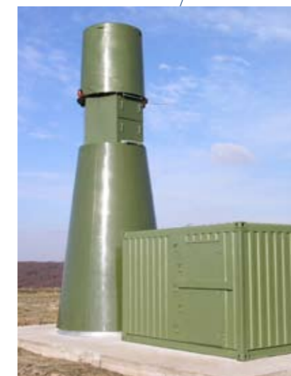
Ground Tacan Installation
